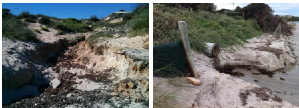
Plate 20: Scouring and erosion stormwater
