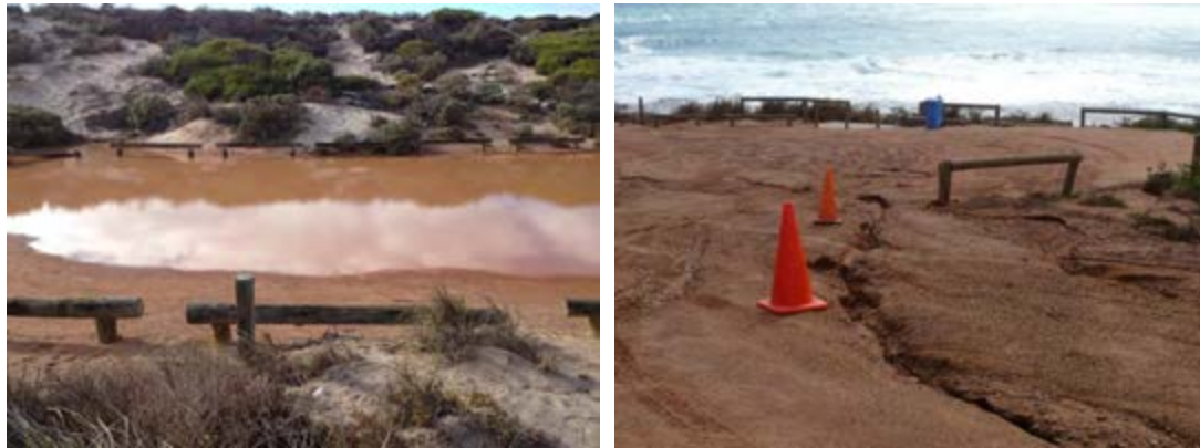
Plate 29: Car park flooding and stormwater damage
