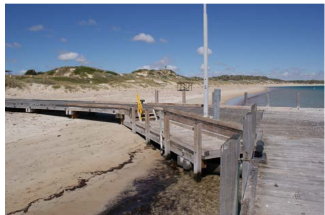
Photo 18: Sand accretion - Port Gregory Jetty (Land Insights, 2016)
