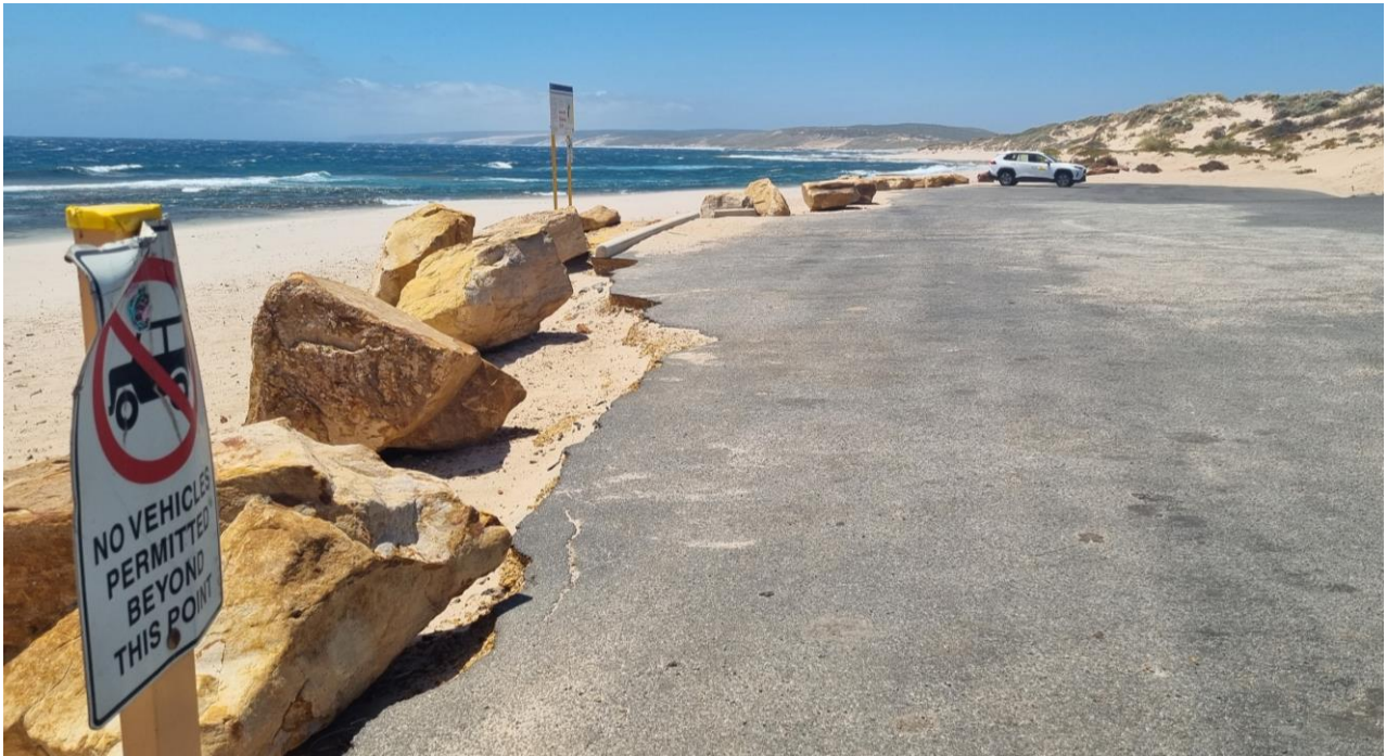
Photo 5 Shelter previously located in front of car park completely destroyed. To be reconstructed in different location.
