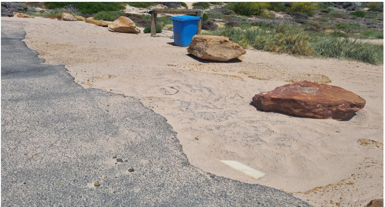
Photo 6 Pavement, gravel and kerb reinstatement required
