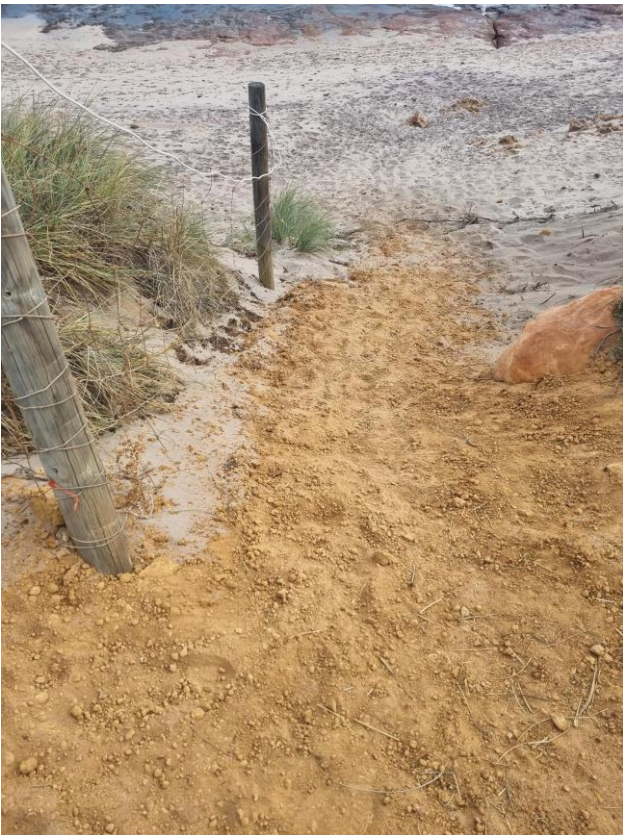
Photo 5 Beach access – temporary works undertaken. Damaged fence and posts to be reinstated
