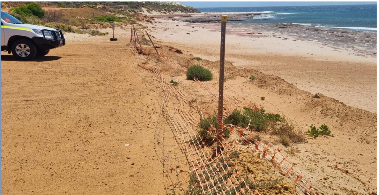
Photo 4 Lower carpark damaged and washed away. New car park proposed to be adjacent to access road
