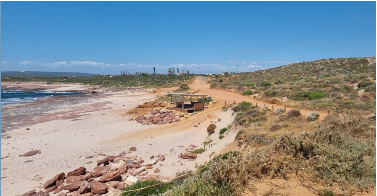
Photo 5 Emergency vehicle beach access damaged. Shelter damaged. Lower car park washed away
