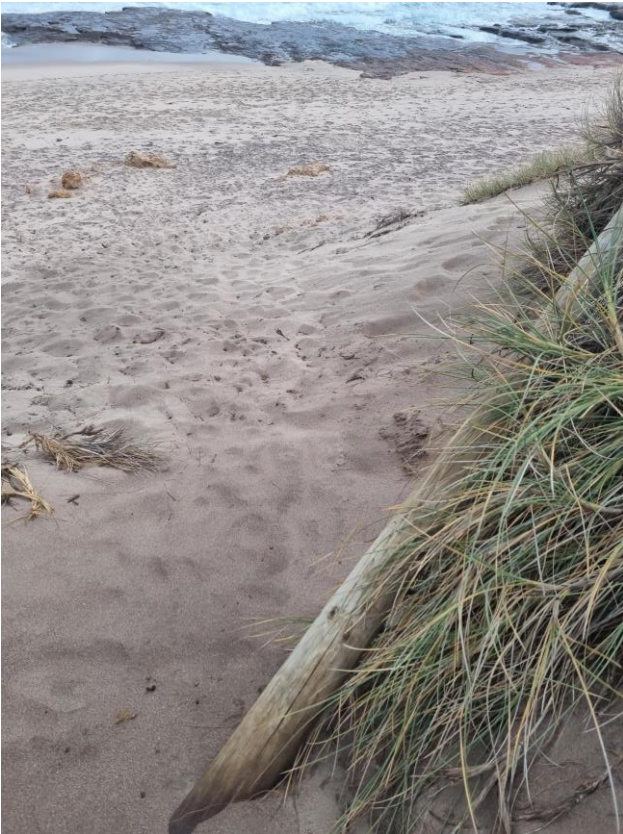
Photo 7 Damaged fence post
