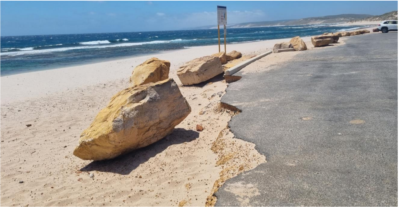
Photo 3 Damaged pavement edge to be cut back, reinstatement of concrete footpath and kerb required
