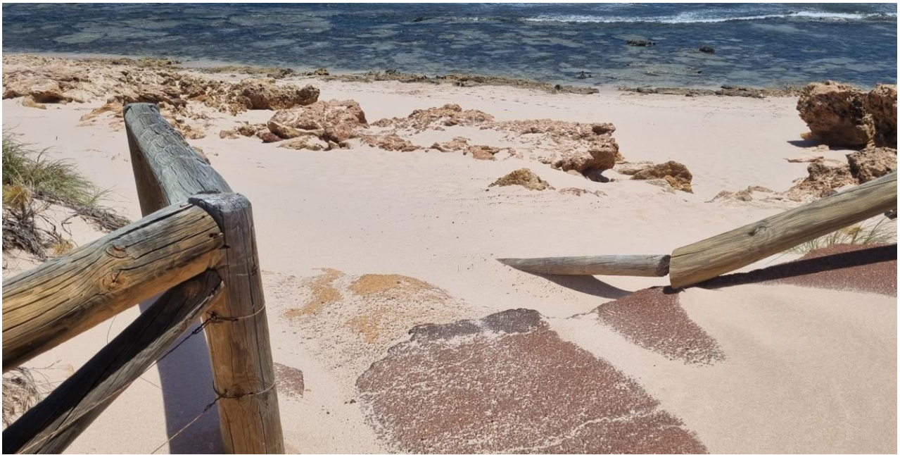
Photo 11 Damaged log fences and beach access to be reinstated.
