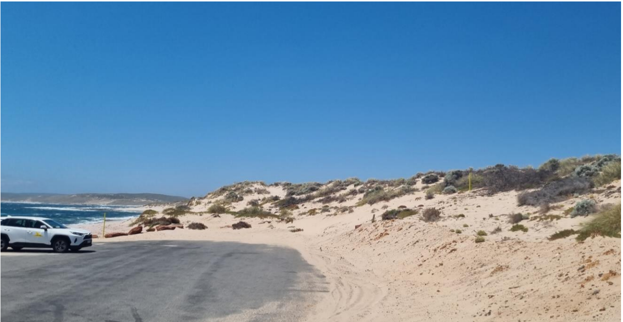
Photo 4 Debris and sand to be cleared off the pavement and dune reinstatement required
