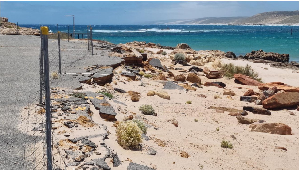
Photo 8 Damaged pavement to be cut back. Rock wall to be replaced with a limestone block retaining wall
