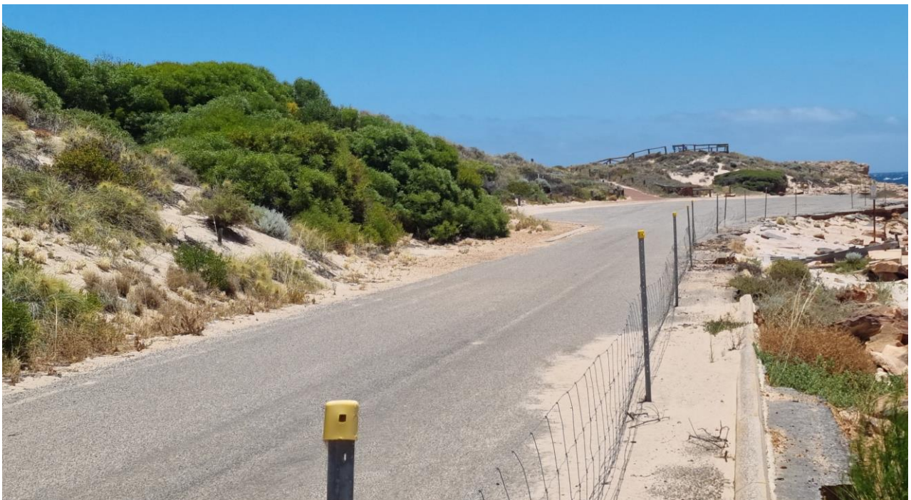
Photo 12 Damaged pavement, rock wall and beach access.
