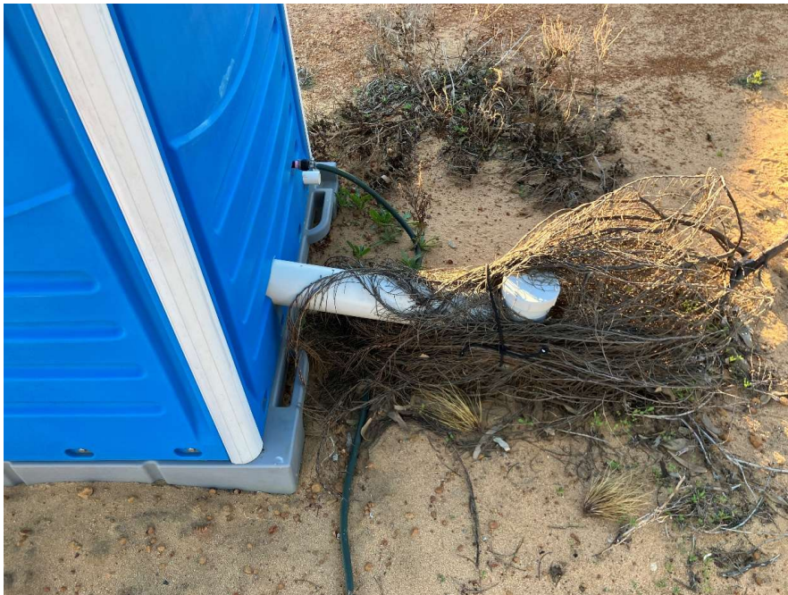
Connection to sewer with dead vegetation strapped to it to disguise connection. Water Supply via hose.
