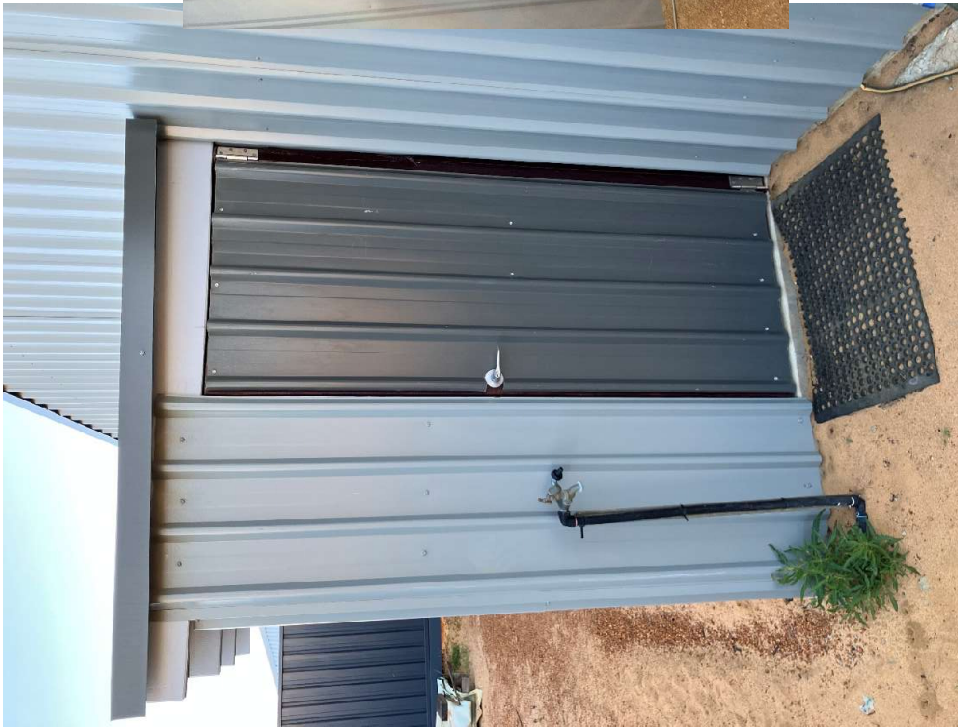
Front of unauthorised addition – Bathroom owner describes enclosed outdoor shower
