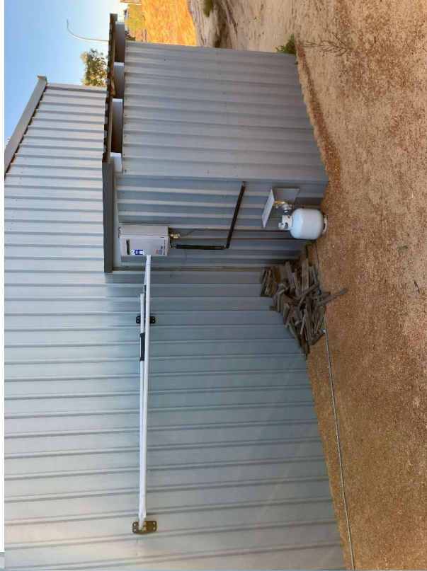
Side and rear of unauthorised extension showing washing line, gas hot water system and gas bottle connection
