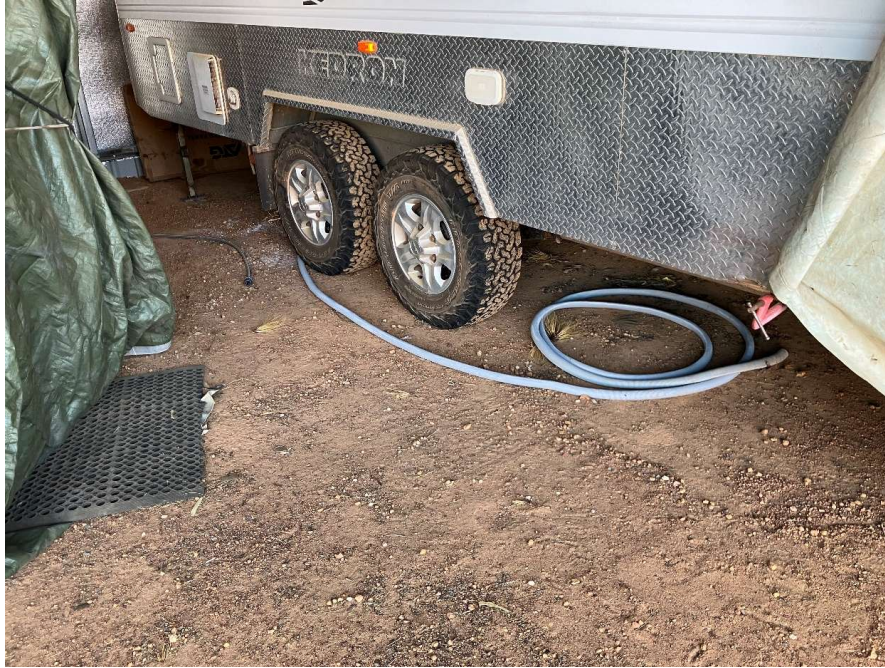
Waste Water pipe curled up under van. Appears to be set up to direct wastewater into grated pit associated with unauthorized wastewater system shown overleaf.
