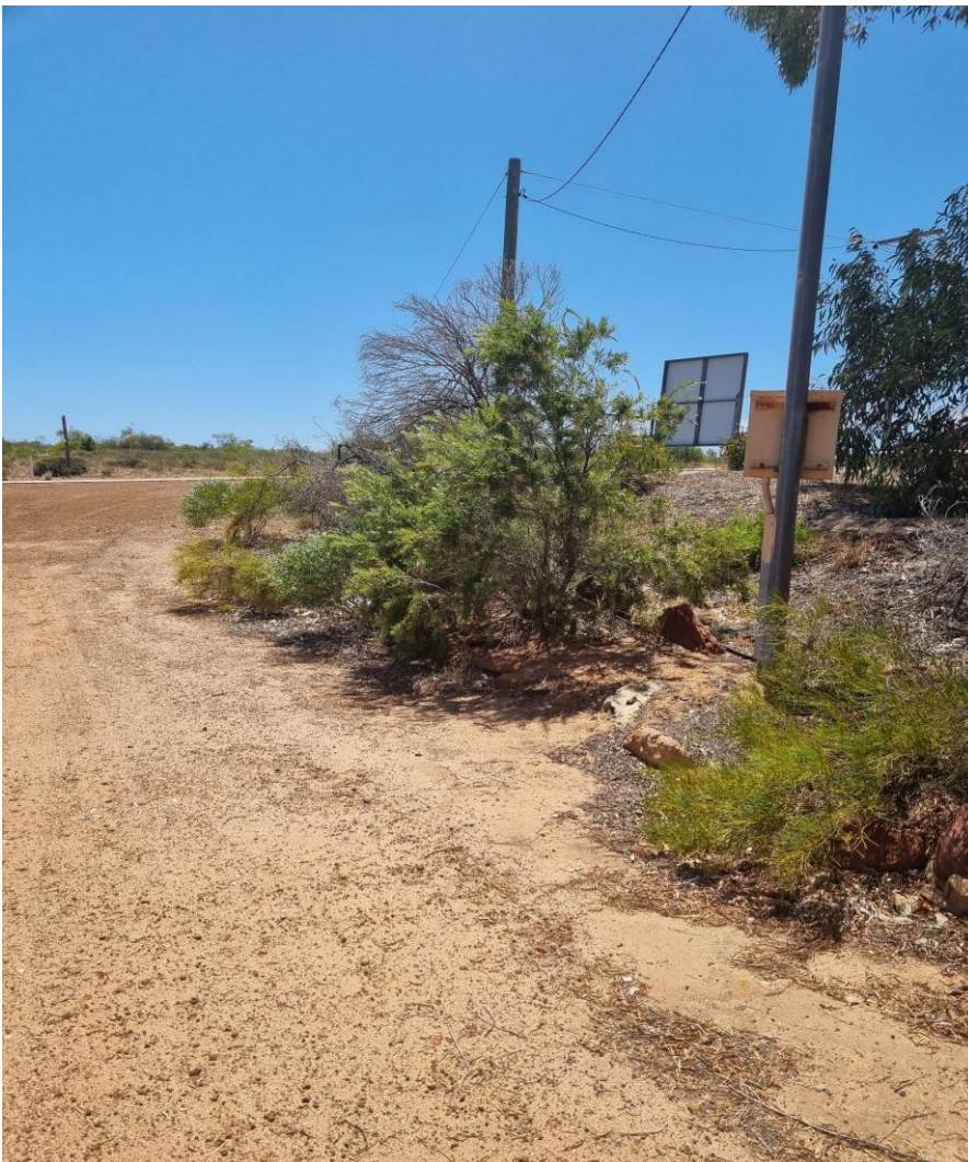
Photo 8 Existing power connection to be upgraded and replaced by Western Power.
