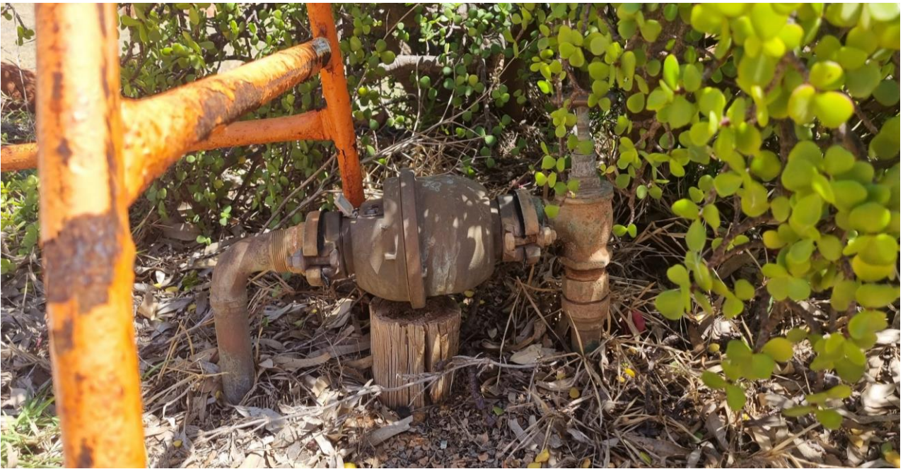
Photo 7 Existing water meter
